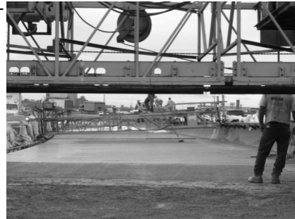
Overlay after spreading. Note finish operation and covering after placement in background.
