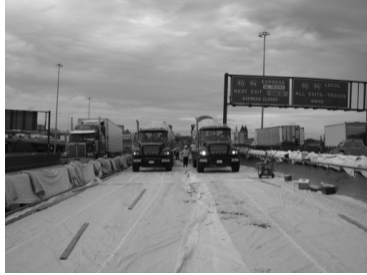
Bridge deck, water saturated, covered. Trucks drive on cover until concrete is placed.
